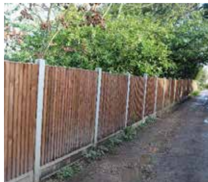
Figure 50 Fences are common in the Conservation Area's periphery, though post and panel fences do not make a beneficial contribution to the character
