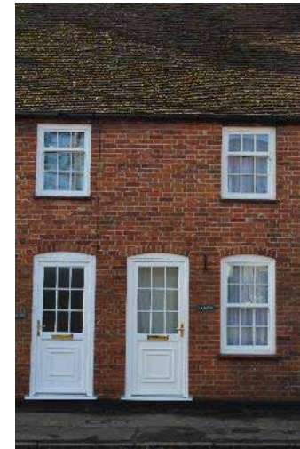
Figure 76 Loss of Architectural Details
